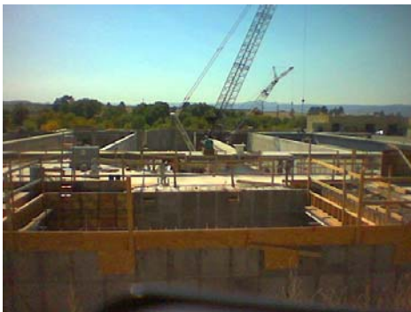
Plum Creek Authority Plant
