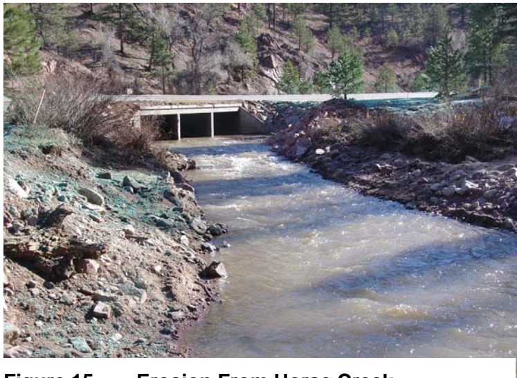
Figure 15 Erosion From Horse Creek
