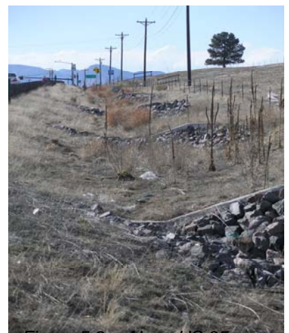
Figure 5-2 – Along US 85, concrete weirs with rip rap reinforcing eliminates hydraulic piping, undermining and erosion
