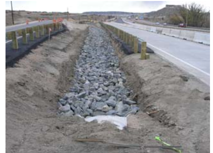
Figure 5-1 – CDOT channel grading along I-25 near Castle Rock assisted to keep approximately 24 tons of sediment out of Plum Creek
