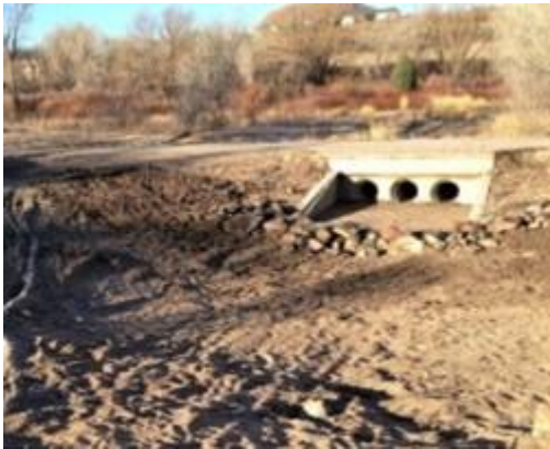
Before: 3-24" Culverts completely filled in with sediment following a June 2015 storm event.
